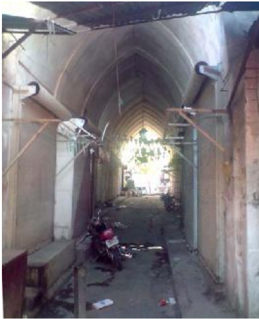
Above left, arched shop entrances are entirely concealed by steelwork when the shops are closed.
