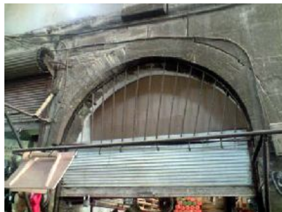
Below , old iron grill closing a fanlight arch in the Deir Ezzor souk.
